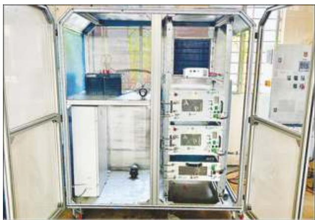
Green Hydrogen Demo Plant installed at VSI
